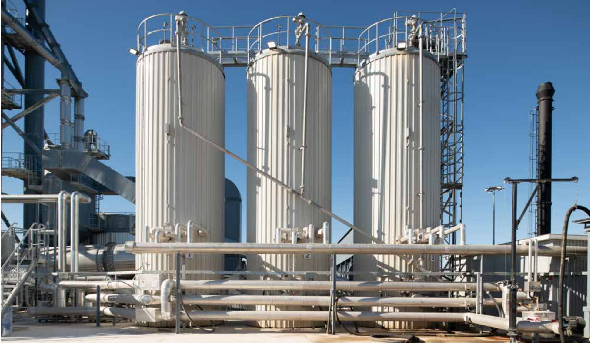
Bitumen Service & Stock Tank
