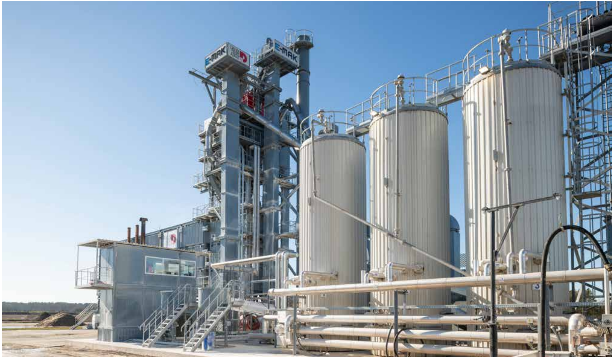
Bitumen Service & Stock Tank
