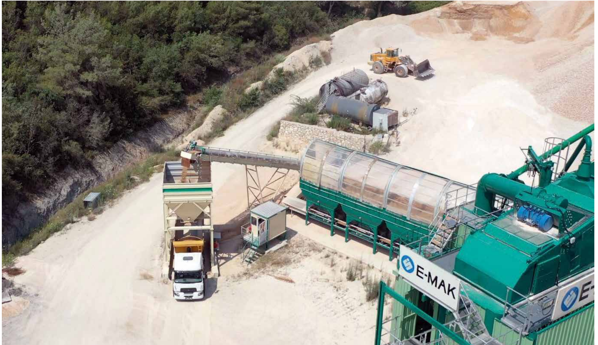
Cold Mix (Mechanical Stabilization) Asphalt Plant
